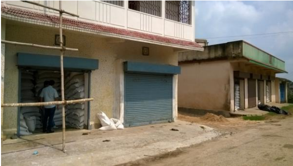
Faulty Feed Godown
